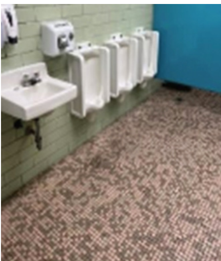
Plumbing fixtures have become a maintenance issue. Repair or replace as needed.
