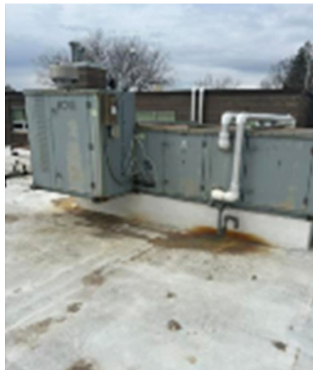
Roof top HVAC unit passed its life expectancy with maintenance issues. Recommend replacement for indoor air quality improvements.
