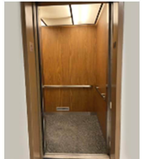
Upgrade elevator to bring up to current codes.
