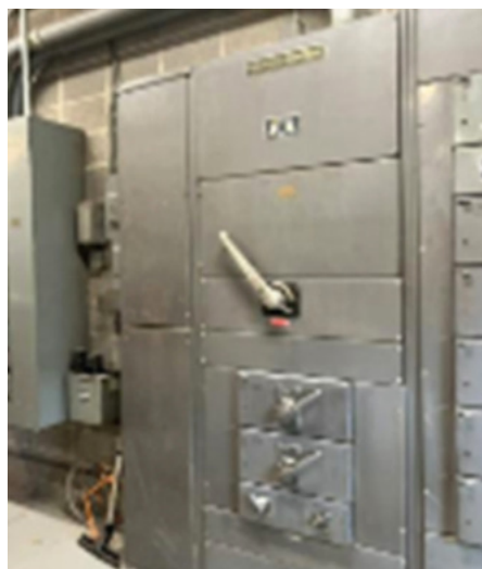
Aged electrical switch gear and panels needing repair and/or replaced as needed.
