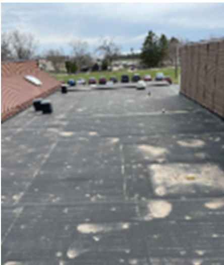
Membrane roof passed the warranty period and showing signs of failure.
